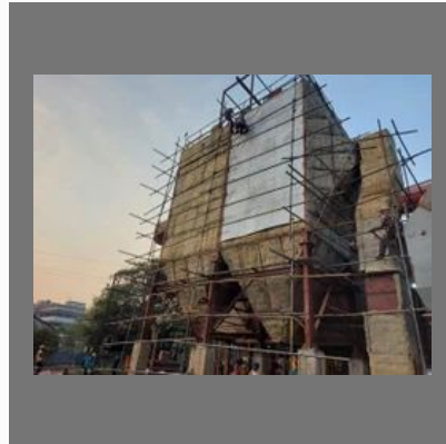
Rockwool Insulation Services
