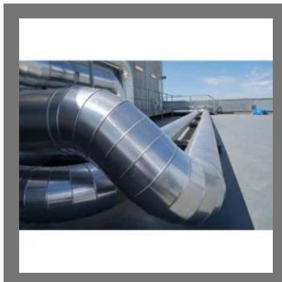
Cold Insulation Services
